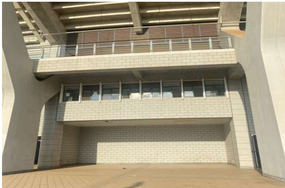
Figure 5. 5: Bingu National Stadium incomplete shop spaces
